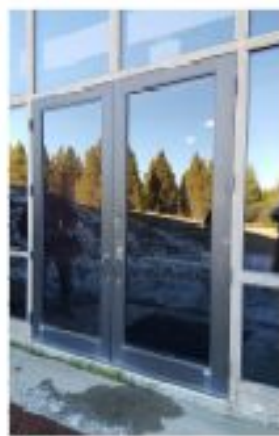
EXTERIOR DOORS - NEED REPLACEMENT
