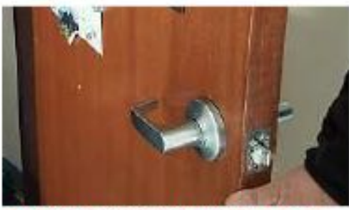
CLASSROOM HARDWARE UNABLE TO BE LOCKED FROM INSIDE ROOM
