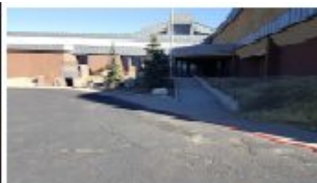
NON ADA COMPLIANT FRONT ENTRYWAY
