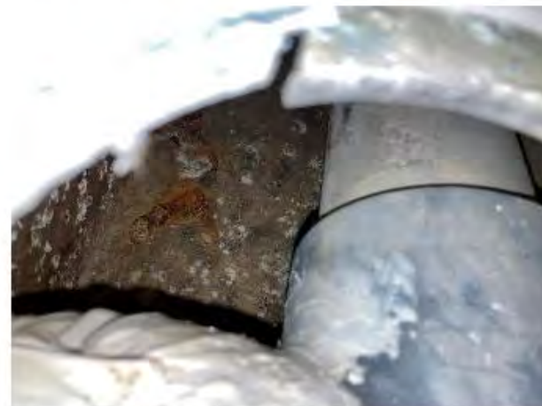
Image 6: Interior Pool Gutter Corrosion/Staining
