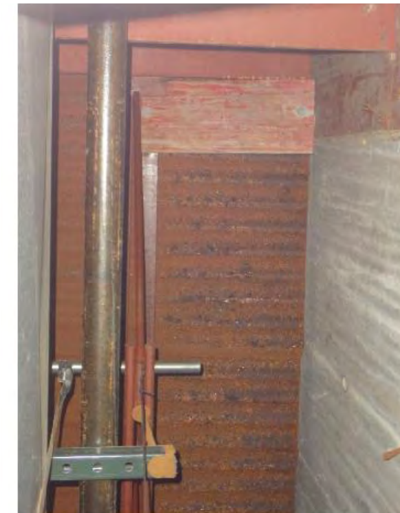
Photo 4: Rust on 2 nd floor deck
