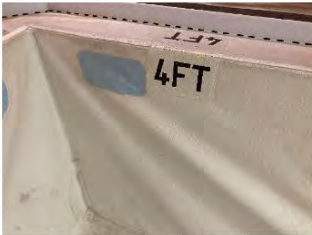
Image 3: Loose/Patched Pool Liner
