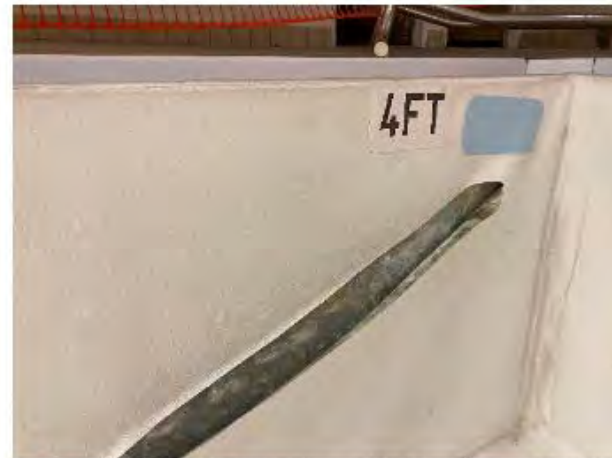
Image 4: Liner Compromise with Aluminum Staining
